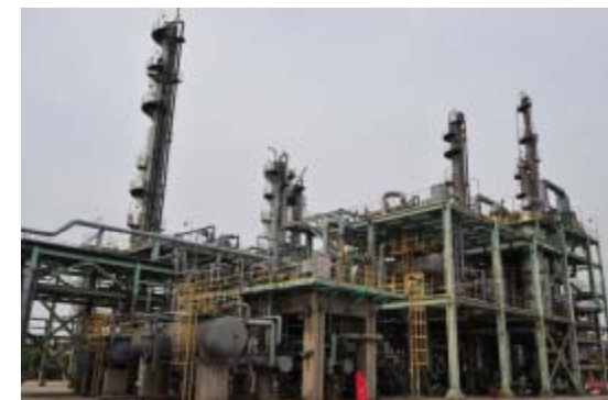
OCC unit in Puyang
