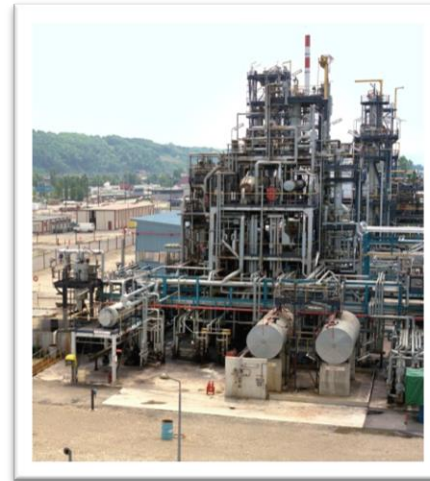
Solvent Deasphalting unit
